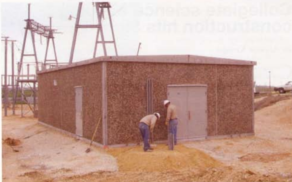
New Braunfels Utility chooses Lonestar Prestress Manufacturing's Easi-Set precast concrete buildings, engineered to withstand 140 mph winds, to house SCADA equipment and other vital infrastructure at local substations currently being overhauled.
