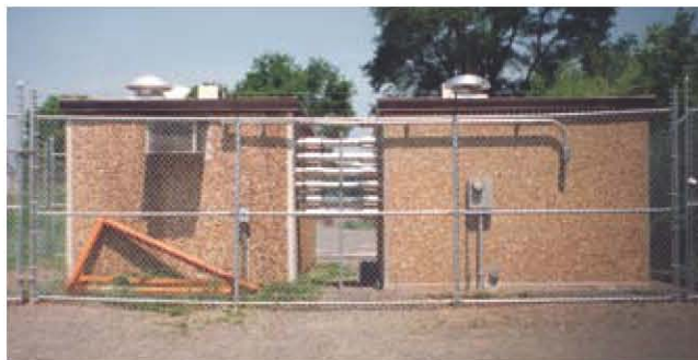
AT&T fiberoptic regeneration shelters, Calverton, VA
